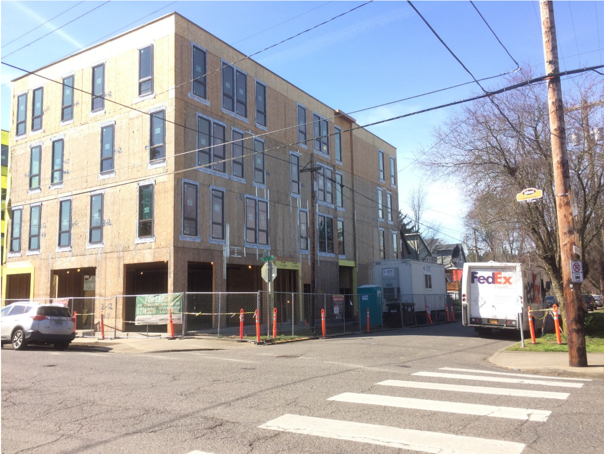
Photo 4. A building façade (in shadow) under construction facing a local service street (SE 13 th and Lambert). More articulation would improve the façade (C2).
